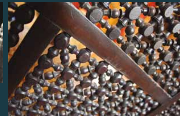
Left: Restoration of the mahogany Moroccan balustrade at the bottom of the Grand Staircase was a major challenge. It had to be taken apart and the damaged or missing individual pieces replicated on a lathe before re-assembly. This was done off-site in the Leicester workshop.
