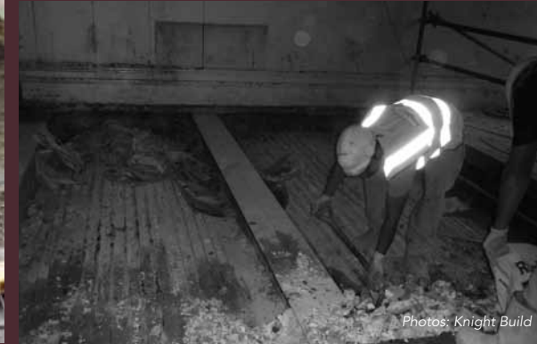
Above: The basement posed particular access and egress problems. Tiny diggers and motorised barrows were taken down and, where possible, mini cranes were situated over shafts, but large quantities of demolition rubble still had to be ‘handballed’ - ie. removed by hand!
