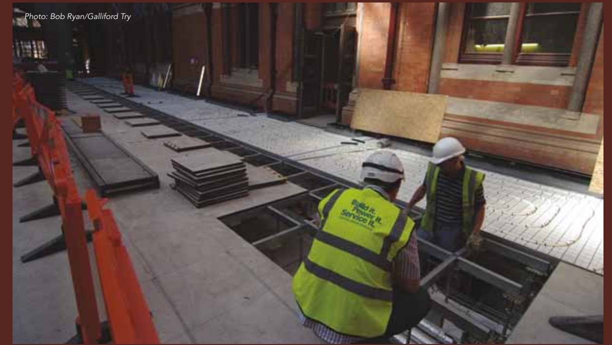
Above: Fitting and assembly of the underfloor heating in the hotel reception.
