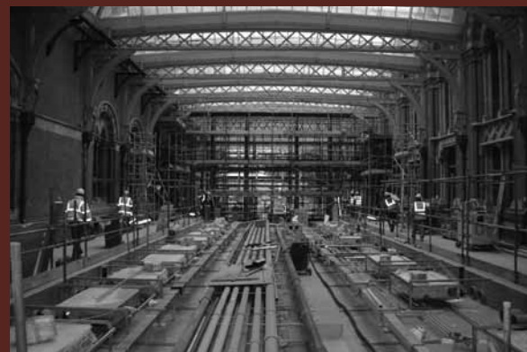
Above: Most of the main services for the hotel and private apartments run under the old taxi-rank, now the hotel lobby and reception.
