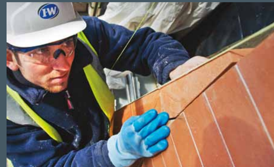
Top: For the hotel's new West Wing, 172,000 Charnwood handmade facing bricks were cut to height by Bulmer Brick. Behind these are 60,000 Charnwood handmade standard imperial backing bricks.
