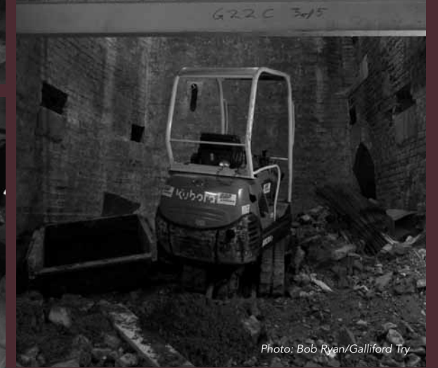
Above: Excavations in the basement were up to 6 metres deep, in very cramped conditions.
