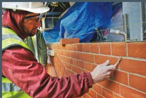
Above left & left: Some of the red rubber bricks had to be cut exactly to size on site. Great care was taken to match the existing 5mm jointing on the facing bricks. Hardwood jointers were made up to ensure accuracy.
