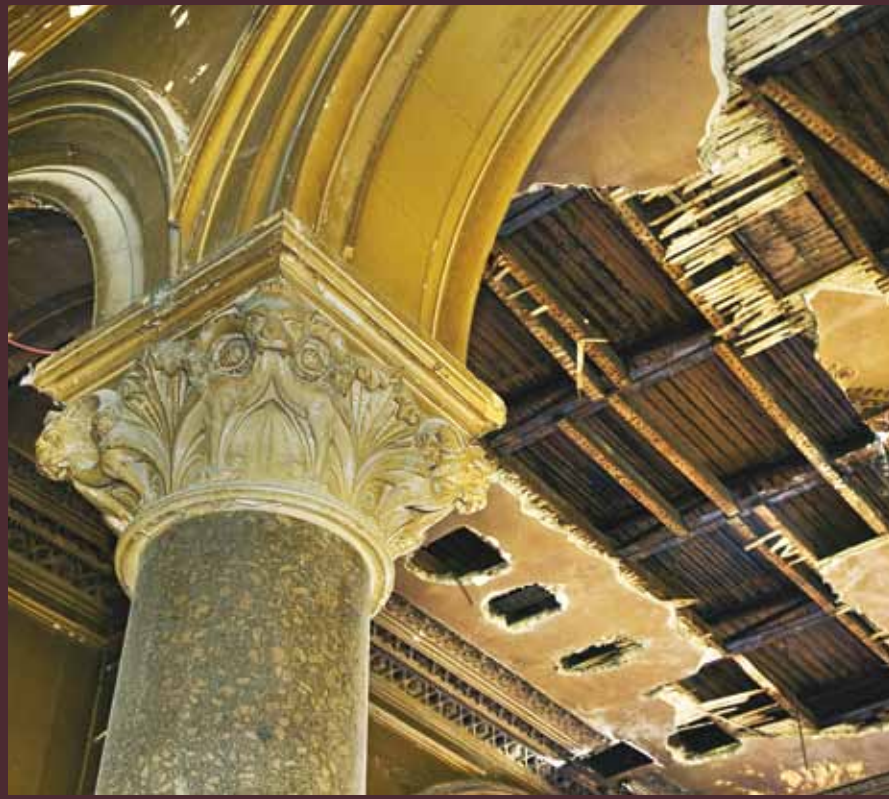
Above: Extensive plaster damage in the Club lounge.
