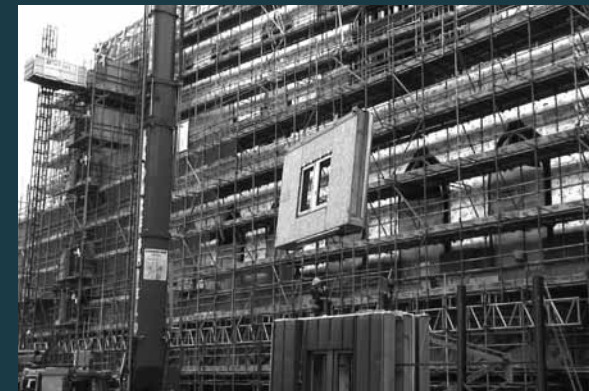
Far right: Due to the method of construction, the joining seams between the panels were slightly wider than the other vertical seams. This created an extra 'feature' that had to be approved by English Heritage as it had not appeared in the original concept.
