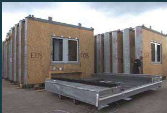
Left & below left: Up to four mansard (roof) or 12 flat wall panels came in at a time by low loader in planned construction sequence. The panels were carefully craned into position over the top of the building, lowered and then secured to the steel frame using a minimum of fixings.
